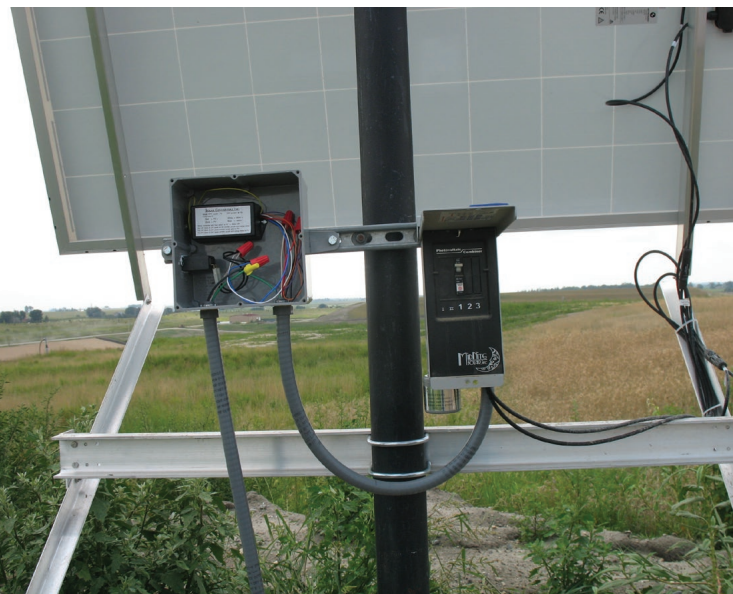
Converter and breaker mounted behind panel
